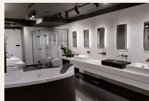
Long illuminated vanity run with mirrors and shower enclosures
